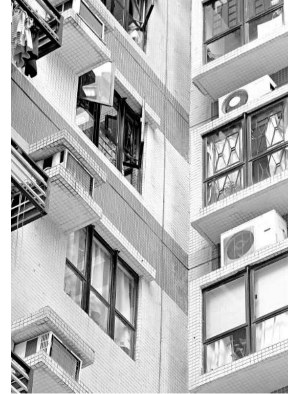
▲冷氣機和相鄰單位太近，熱氣可吹入鄰居屋內
