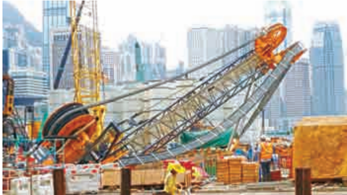
▶灣仔會展地盤內一部重型吊機傾側
