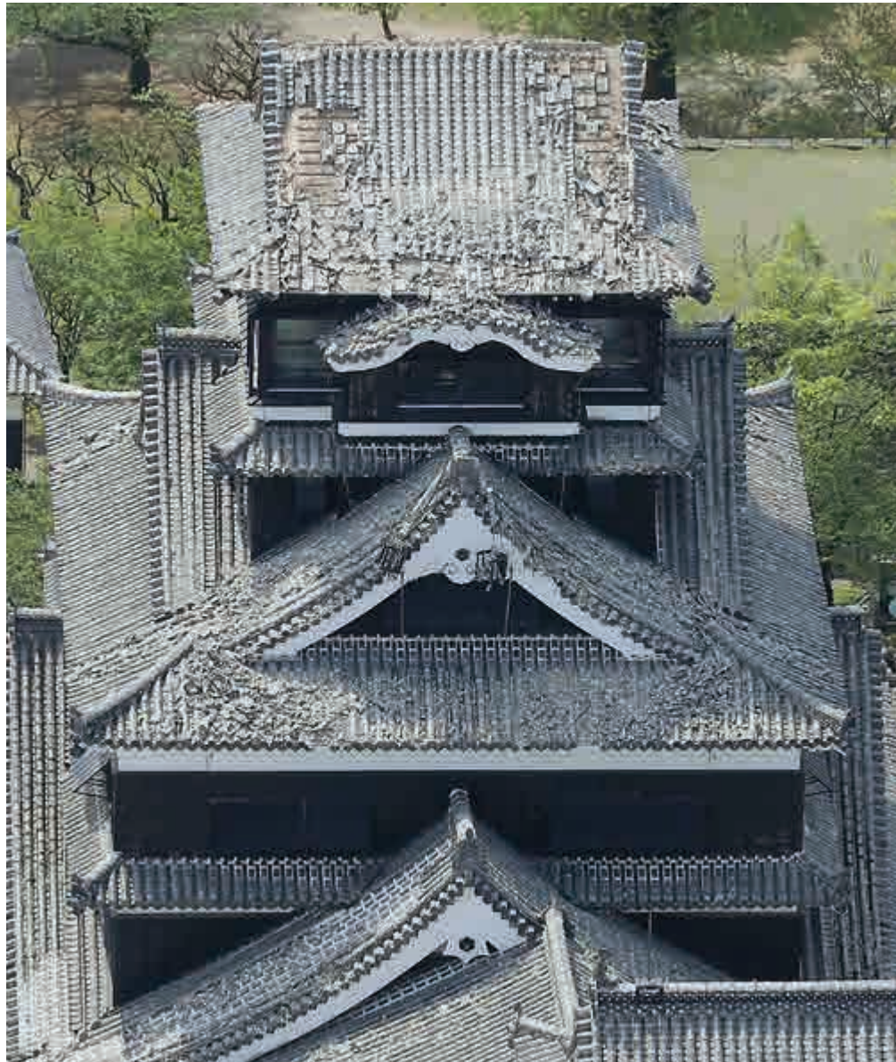
▶熊本城內建築屋頂有多層瓦片垮塌
