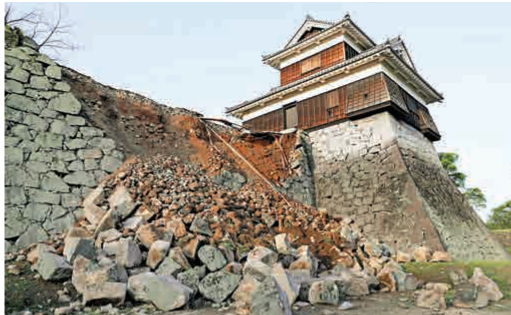
▶熊本城內至少有6處石牆崩塌
